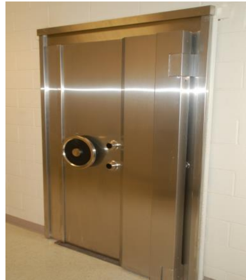
Each vault is accessed via a Level 5 secure and fire resistant vault door with at least a 4-Hour UL Rating of at least 350.
